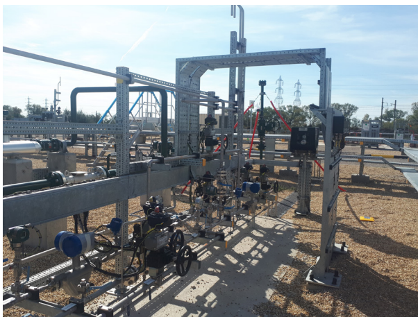
KROHNE Coriolis mass flowmeters installed at P2G demonstrator
